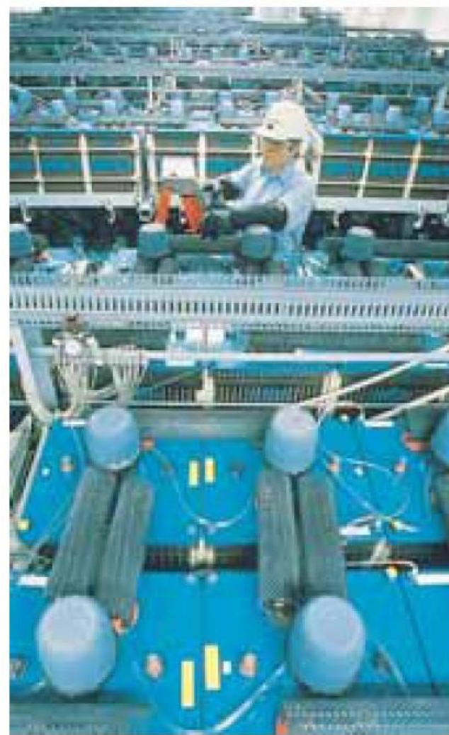
The world's largest battery energy storage plant (dismantled in 1996) connected over 8000 large lead-acid batteries in 8 strings at 1000 V each with a capability of 10 MW of power for 4 hours. Charged up at night, the batteries were then put to use during peak power demands on the electrical system. (Courtesy Southern California Edison Company)
